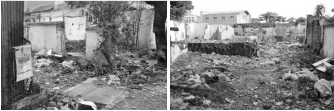
Figure 2. Demolished Buildings Around Cihampelas Area Bandung City. [Source: Author, 2023]
